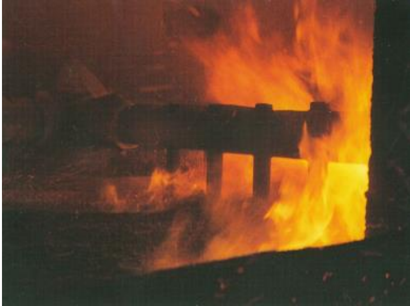
Inside of incinerator
